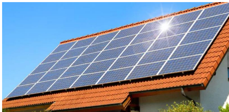
Figure 7: Picture of solar panels on a roof [14]
